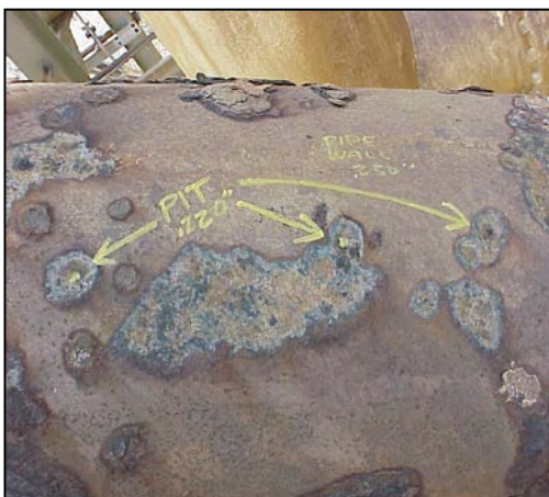
Fig. 2 – Surface preparation as shown is generally unacceptable. In cases where the pipe cannot be properly cleaned, it should be noted that the final ultimate properties of the composite layup may be compromised (such as bonding to the steel surface).
