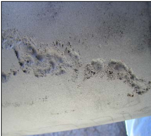
Fig. 1 – The sandblasting done on this line revealed more damage than was visible during the initial inspection. Proper cleaning is essential to a sound repair.
